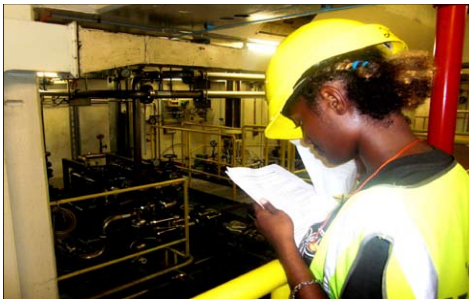
Sandra Amet referring to her notes while at the Mechanical room at Rouna 2
